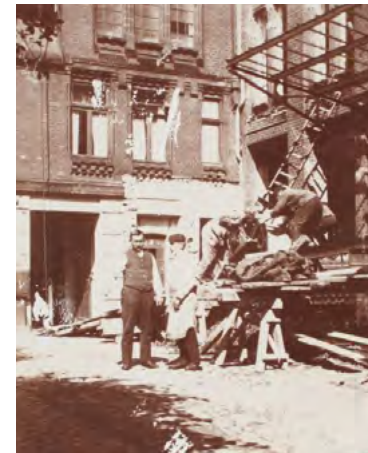
Left: Courtyard with loading ramp for deliveries Above: Building the ramp; both photos from 1909
